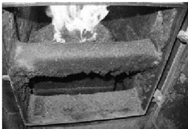
Fig. 13 Very dirty combustion chamber.
