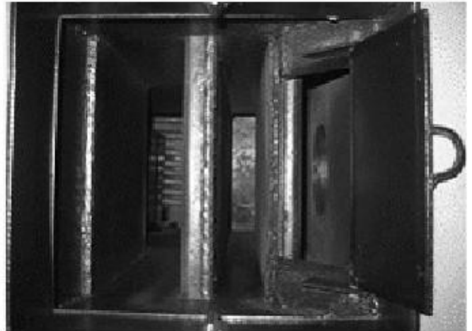
Fig. 16 Very clean boiler exchanger
