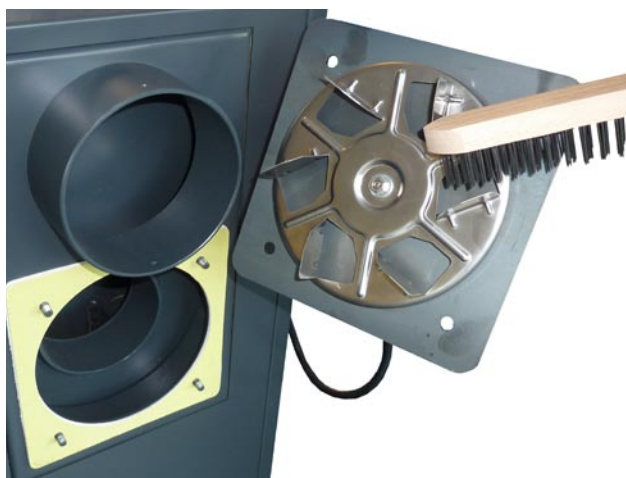
Sample cleaning of impeller and checking uprightness of vane on exhaust fan (boiler D31P)
