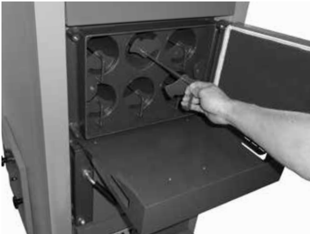
Cleaning of the boiler's tube exchanger using the built-in waste gas decelerator
