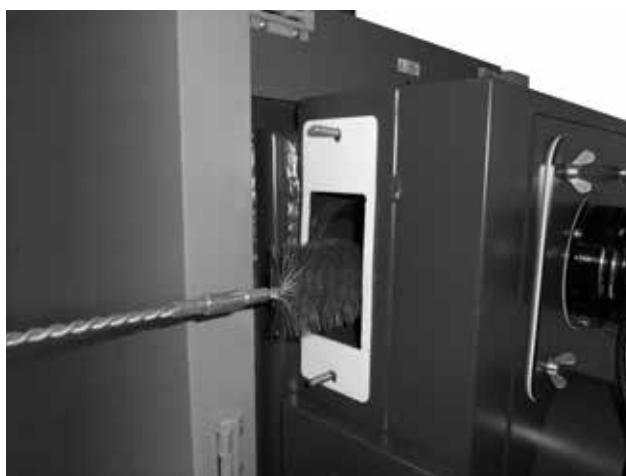
Should be done after the tube box above the boiler's combustion chamber had been cleaned
