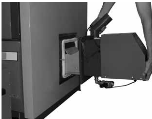
Burner removing for year servicing and cleaning
